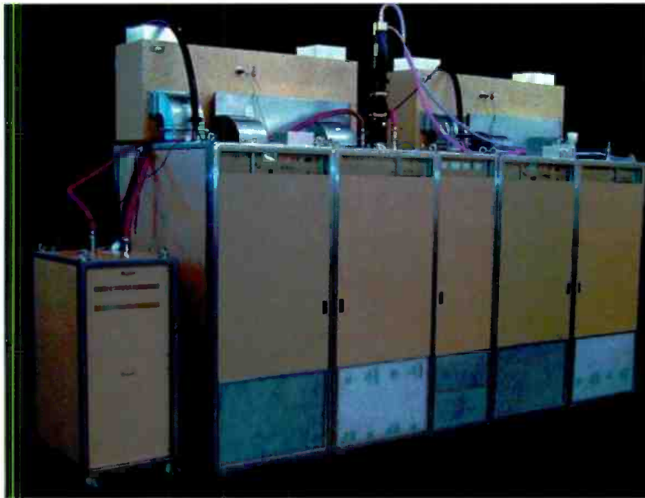
Helco's 50kW IOT transmitter for DTV applications offers two tubes and two 90kW switch-mode power supplies.
